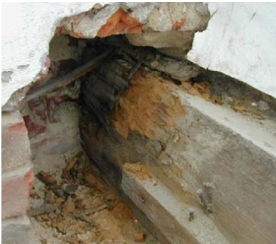
Wood rot of wooden floor beams
